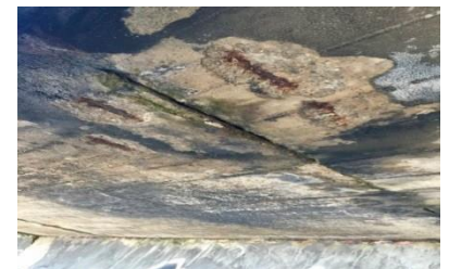
Extent of the chloride induced corrosion
