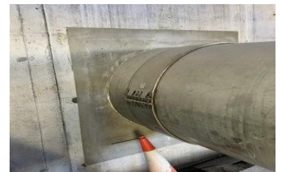
Large stainless steel pipe
