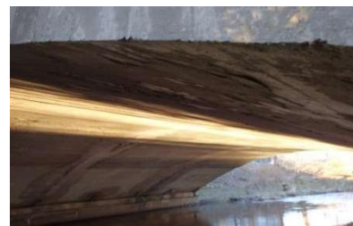
Spalling to arch.
