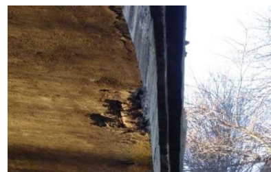
North arch ring mid span spalling.
