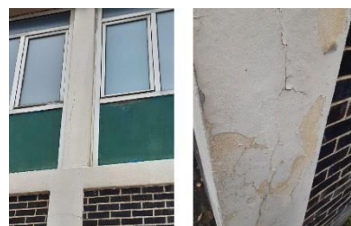
Left: typical cracking to the concrete. Right: Failure of existing coating
